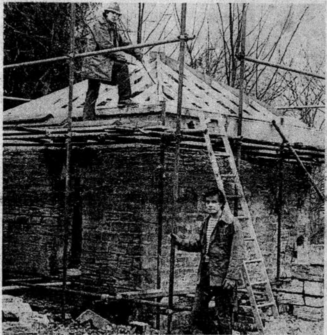
Peter Sanderson at work on the roof of the dove-cot with trainee Dominic Devoy. (W1076).
